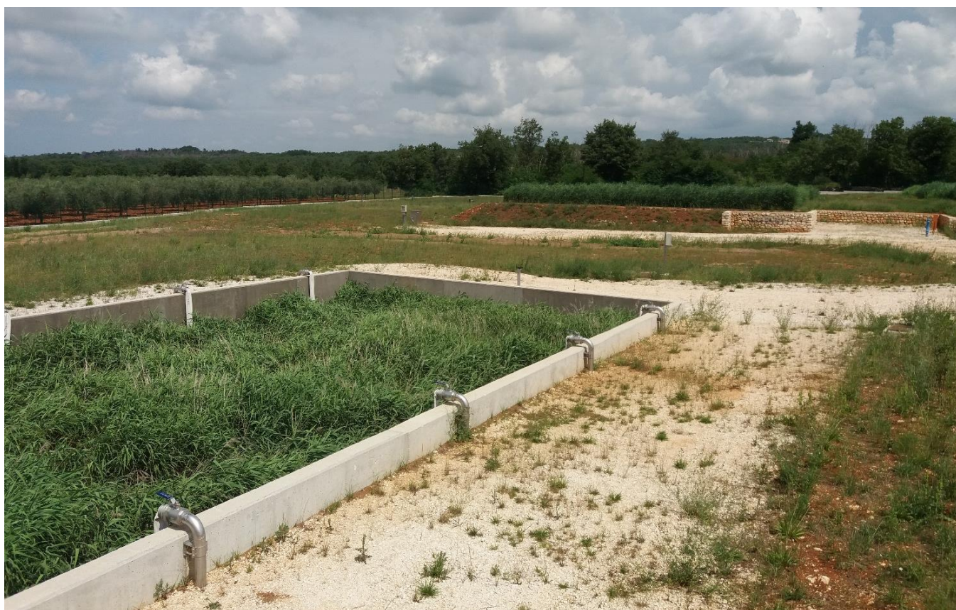
Figure 13: RB (front) with one of the five beds of constructed wetland (back) in Kastelir
