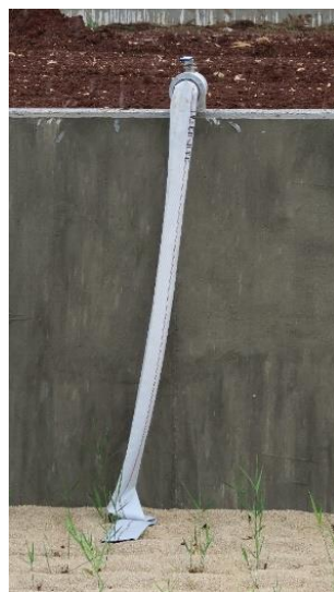
Figure 8: Sludge distribution pipe
